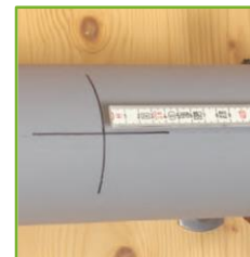
04. Minimum distance between two Saddles must be 300mm*, this is also the rule between saddle and other types of welding.
