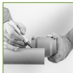
03. Mark the correct insertion depth for the electrofusion fitting on the service pipes. Insertion depth is indicated on the fitting.
